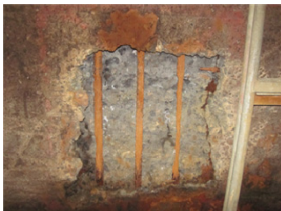
Photo 1 Corrosion of rebar
