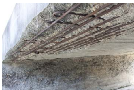
Photo 2 Slab bridge damaged due to concrete neutralization
