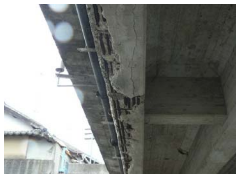
Photo 3 RCT-beam bridge with salt damage
