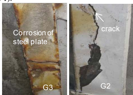
Photo 1 Deterioration on Underside of Girder
